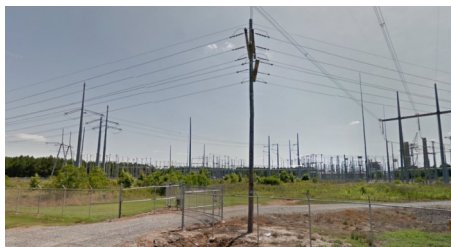
Switchyard outside Ouachita power plant.
